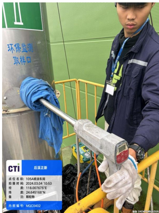
105A 喷涂车间废气排气筒
